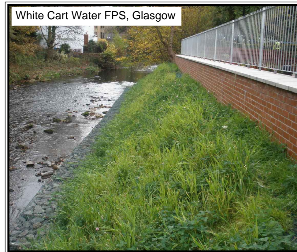
Facing brick finish with precast concrete coping stone and galvanised railings. Reinforced earth embankment and gabion basket toe armour.
