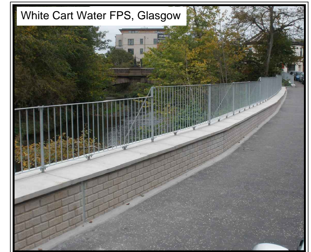
In situ concrete - brickwork type form liner finish with precast concrete coping stones and galvanised railings
