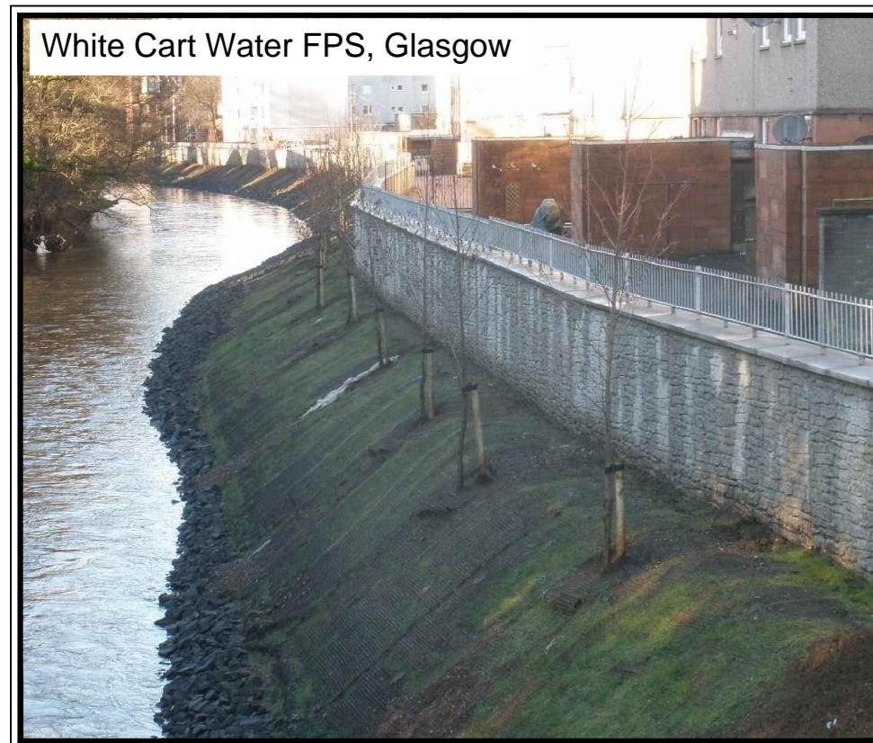
In situ concrete - stone wall type form liner finish. Also shows reinforced earth embankment at early stages of vegetation growth.
