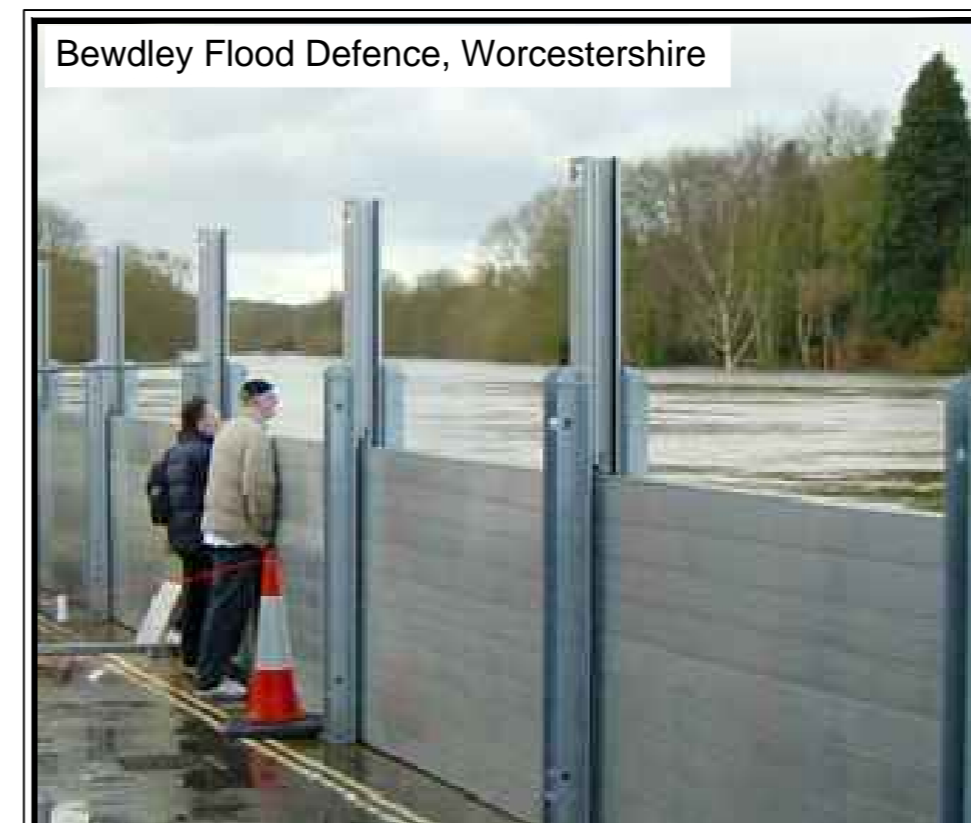
Demountable flood protection - could be used in combination with solid lower defence wall to increase flexibility in the future
