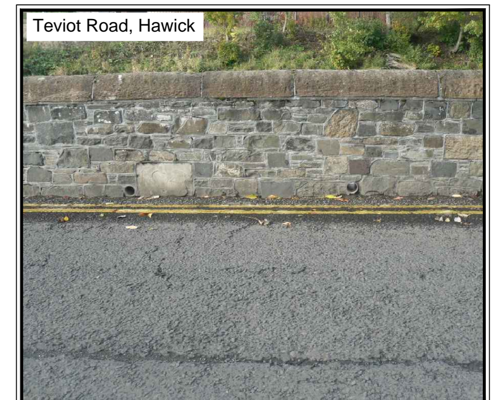
Stone clad masonry wall on Teviot Road - propose to re-use existing stone as cladding to new flood defence wall
