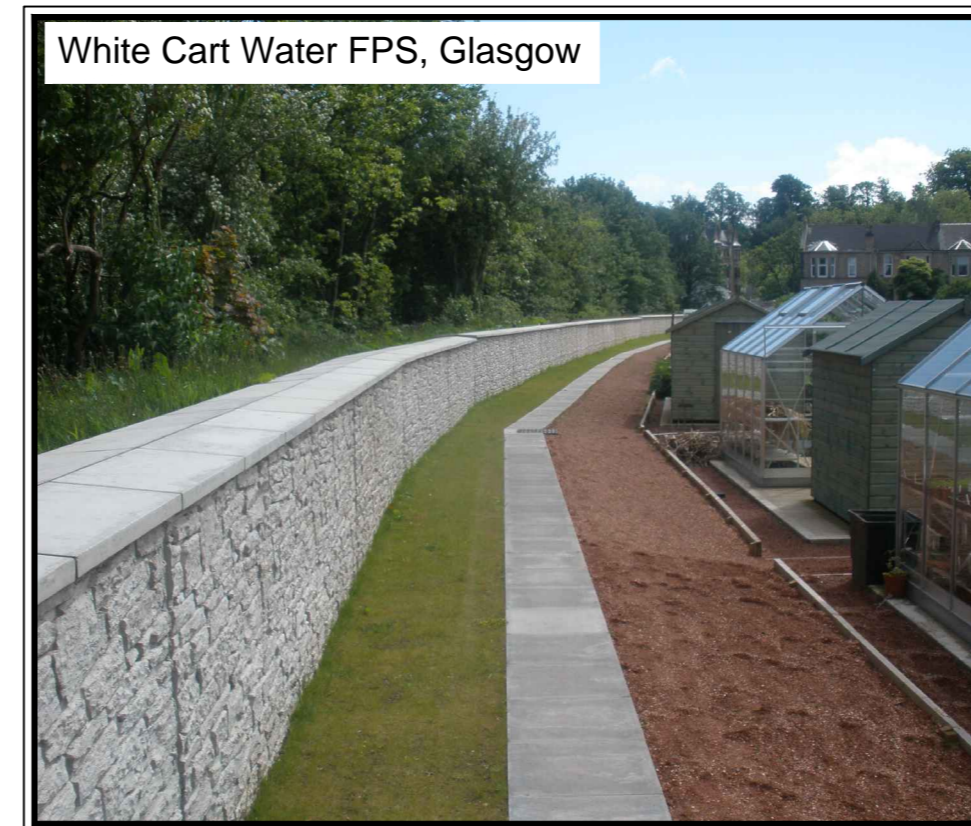
In situ concrete - stone wall type form liner finish with precast concrete coping stones
