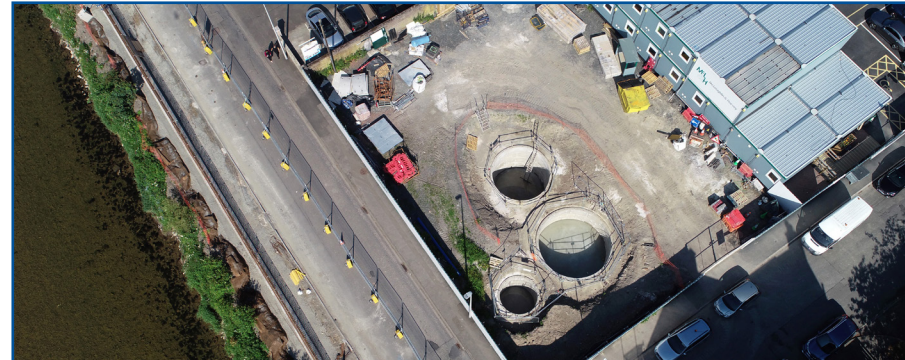
Eastfield Road pumping station consisting of valve chamber, bauer chamber, wetwell and associated pipework awaiting concrete slabs and mechanical kiosks to complete
