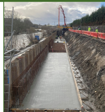
Lower Mansfield Road concrete pours for the base of the L-shaped foundation.
