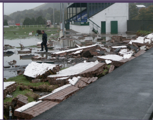
The boundary wall at the Hawick Rugby Football Club fully collapsed following the impact of the flood waters in 2015.
