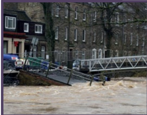
In 2015 high water levels caused a section of the road to collapse into the river on Clebe Mill Street.
