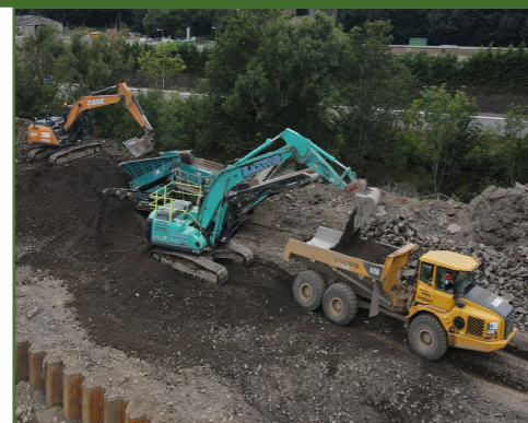
Weensland major earthworks for the flood protection embankment built over the concrete flood wall.
