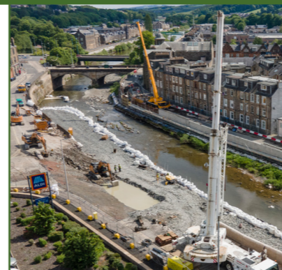
Commercial Road gravity flood wall construction to improve carriageway of A7 trunk road.
