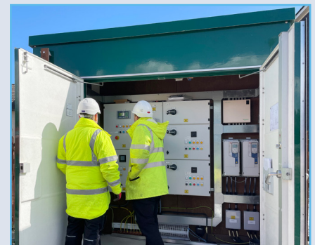
Mechanical kiosk monitoring during commissioning
