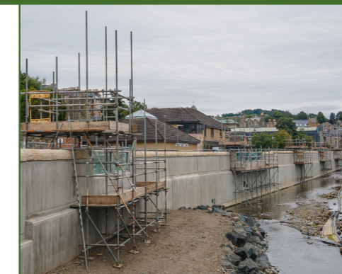
Scaffolding erected to facilitate the testing of the glass panels along Teviot Road by specialist contractor.
